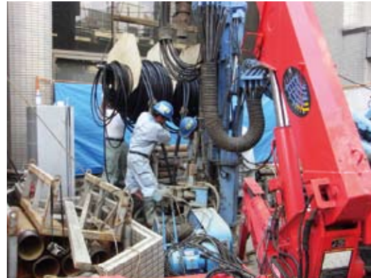
Retrofit of GHP system to an office building in central Tokyo: inserting U-tube (Sasada Building)
